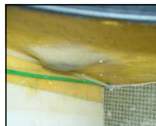
Example of pipe routing through bulkhead immediately below deck
